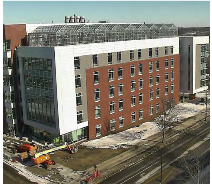
View of construction of ATRB from Science II. The building is located on the northwest corner of Pammel Dr. and Stange Rd., just east of the Insectary building.
